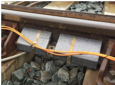
a) Insulation tight against the rail temperature sensor
